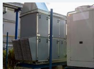
Air Handling Units
